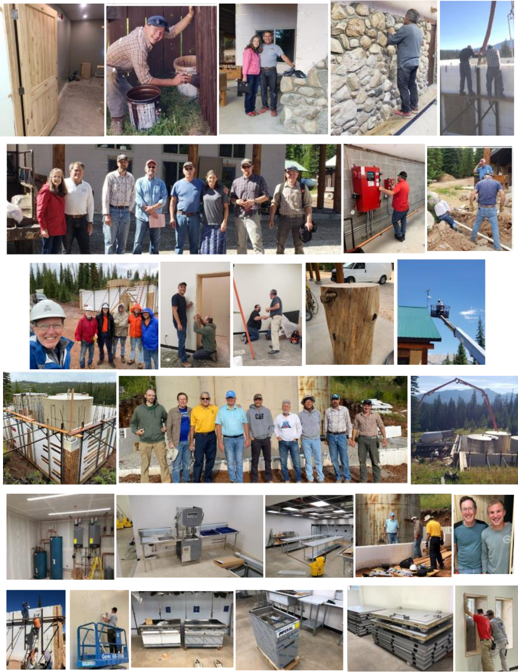
August - Sound equipment installed, fire suppression system made functional, — inside doors set, downstairs bathroom stalls made useable, front rock wall of — south end of Lodge stairwell laid, and many more things!
