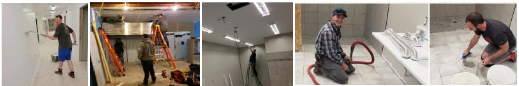
— July - Work on the tank building foundation, Lodge lights inside completed, outside lights set, continuing of tile work, and the kitchen hood set —
